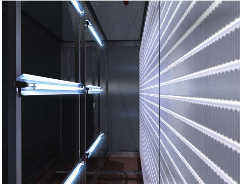
CCX 2X3 Array System Rack-mounted on Cooling Coil
